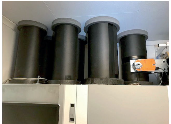
Cellular rubber insulated steel ducts
